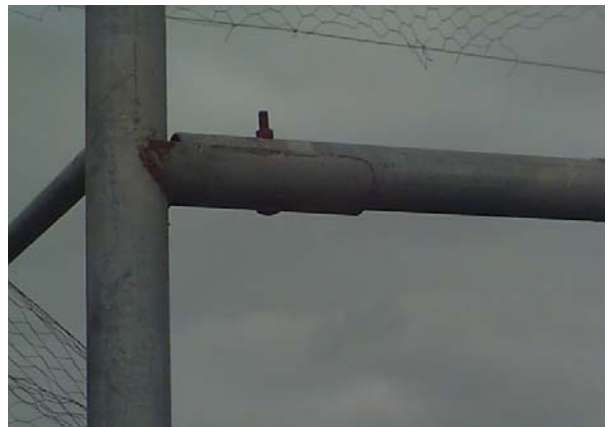
GAA goal - weld and bolt are rusty on the cross bar.
