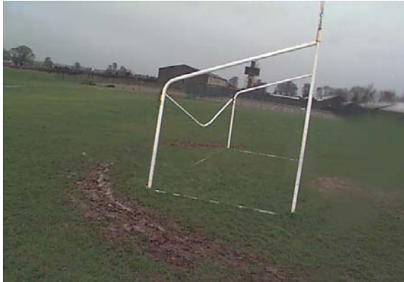
GAA goal frame - frame not sufficiently rigid, back tie bar sagging
